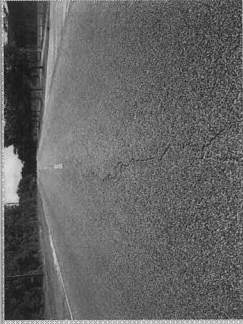
SE 43 rd Street, Paved 1979
